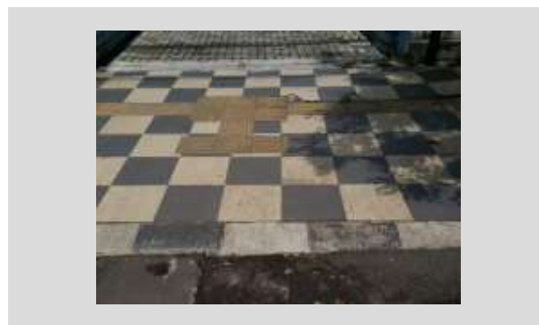
FIGURE 9. The guideline which is located on the ramp is still in good condition and the ramp has a height according to the provisions.
