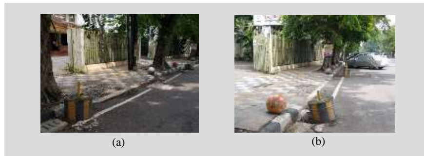
FIGURE 6. (a) Condition of damaged ramp. (b) The condition of the ramp which is damaged and not repaired.
