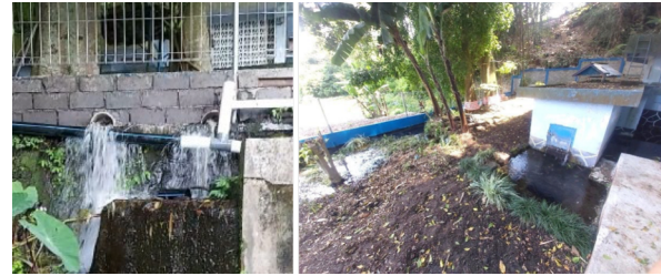
Figure 5. Water intake point outside the small PDAM facility
