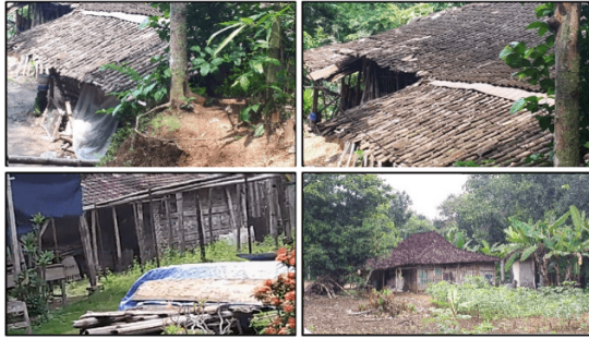
Figure 6 Condition of Houses with Heavily Damaged Category (Source: Observation, 2020)
