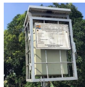
(2) Telemetry Open Standpipe Piezometer 7
