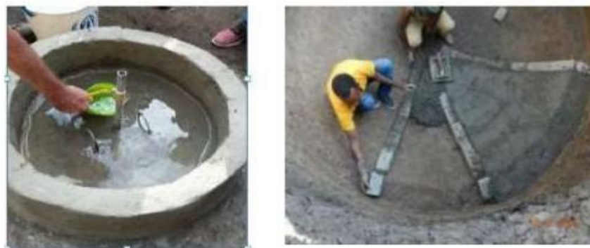
Figure 11. Top of digester filled with water (left), bottom of biodigester (right)
