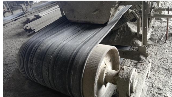
Figure 3. Conveyor belt that does not own safety from outside
