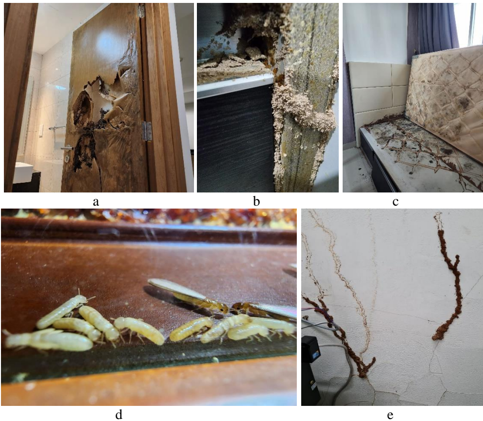
Figure 1. a. Damaged wooden door due to attack by C. curvignathus b. Door frame damage due to attack by M. gilvus c. Damage to the painting frame due to attack by C. cynocephalus c. M. in-spiratus nests are an indication of termite attack activity
