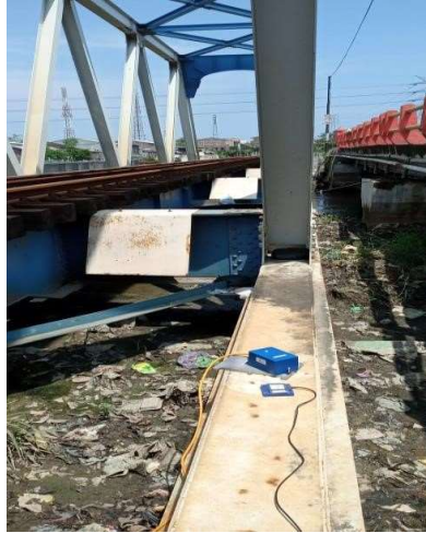
FIGURE 2 Sensor accelerometer placed at the bridge's structure with X facing the east.
