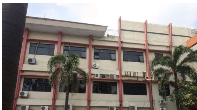
FIGURE 8. The exterior view that could potentially cause a fall hazard
