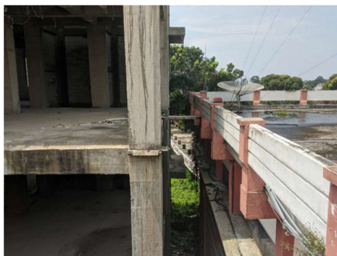
FIGURE 7. The distance between dr Soebandi’s hospital with the new building is 1.87 m
