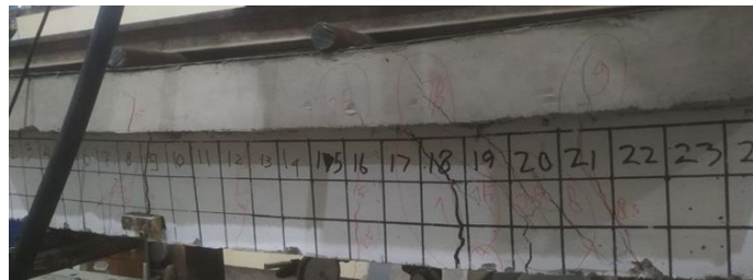
FIGURE 8. The crack pattern of the T-beam
