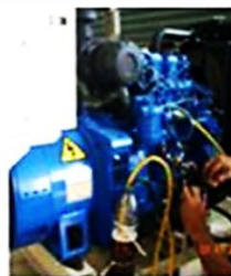
Figure 1. The engine used in this study is the Perkin P135-4 diesel engine with three cylinders with a power of 13.5 HP and is installed on the generator set.
